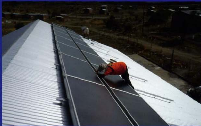
The mounting plates were correctly installed to ensure that the waterhouse would run efficiently.
