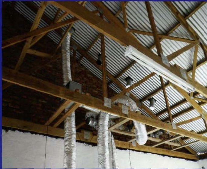
Ventilators from the rows of collectors
